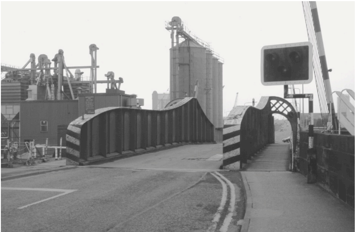
A general view of the bridge from the road on its southern side.
