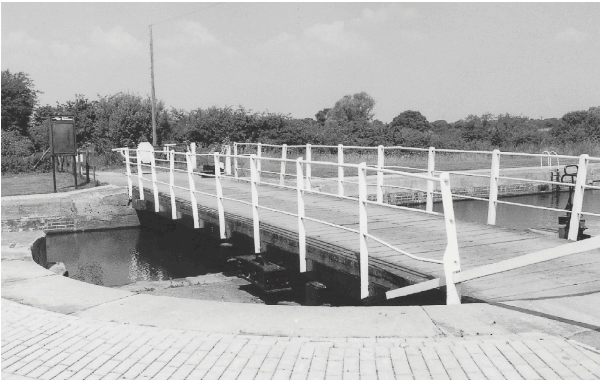
A simple steel swing bridge over Sykehouse Lock on the New Junction Canal. Design work for this canal was carried out by the Aire & Calder Navigation, so reflects their working practice.
