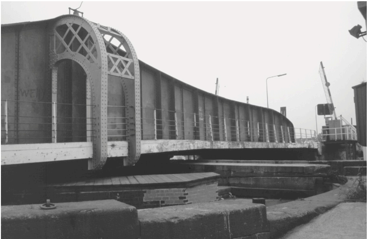
South Dock Bridge seen from the north west. The hydraulic pump is situated in the building on the right of the picture, the operating platform being behind this building.
