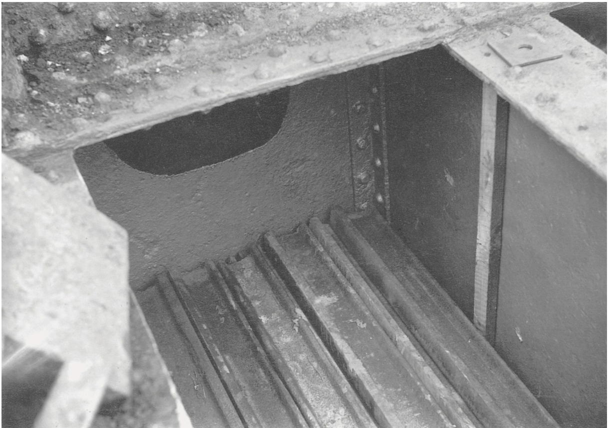
The new ballast inside the ballast box at the tail of the bridge. This extra weight ensures that the bridge does not tip whilst being swung.
