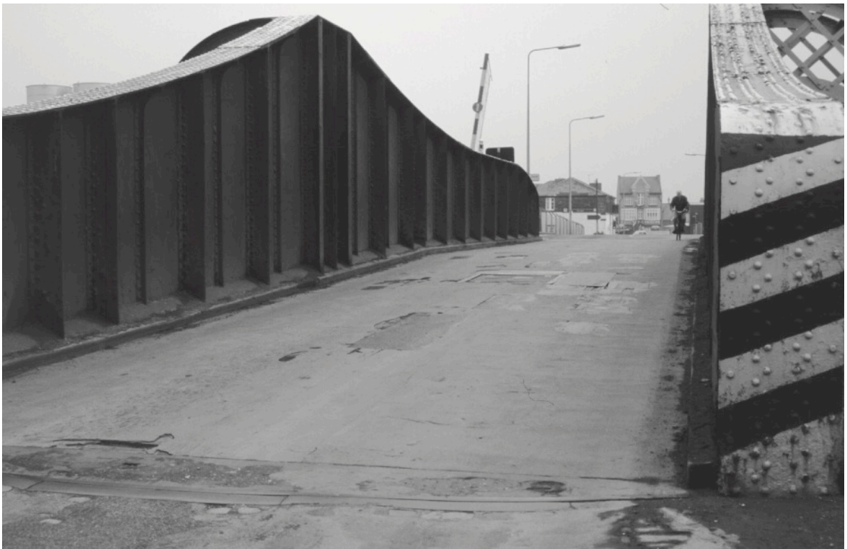
The roadway from the north in 1999 showing the wearing surface applied to the wooden deck covering.
