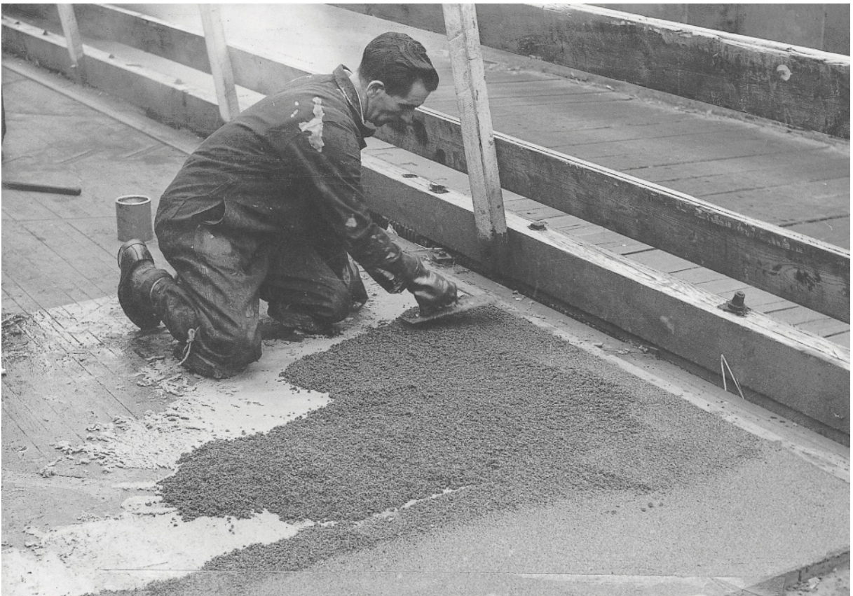
The non-slip wearing surface being applied to the new deck planking, June 1960.
